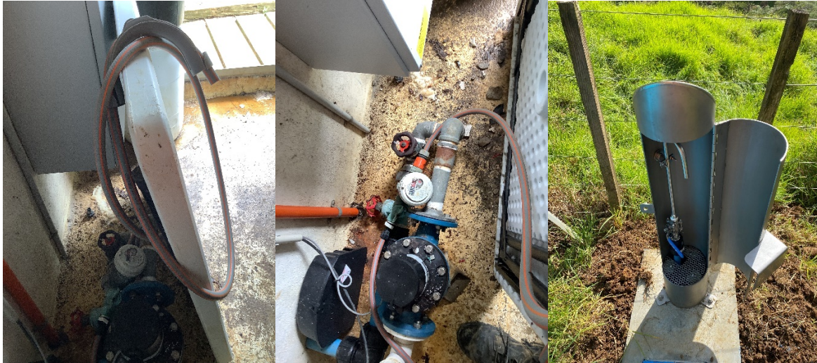
Figure 2. Left - Inadequate and unused WTP sample point, Right – New bollard.
