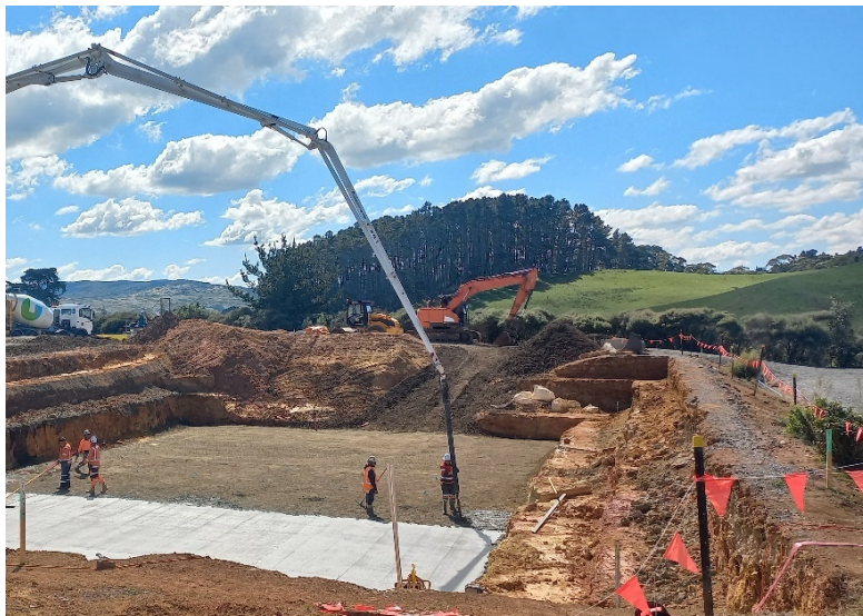
Raglan WWTP MBR Upgrade– Reactor tank site concrete pour, base slab reinforcing will follow.
