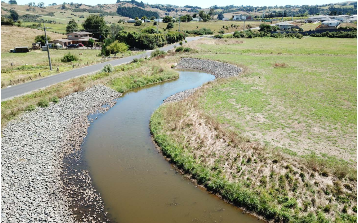
Upstream end of stream diversion. The existing live stream can be seen upper right.
