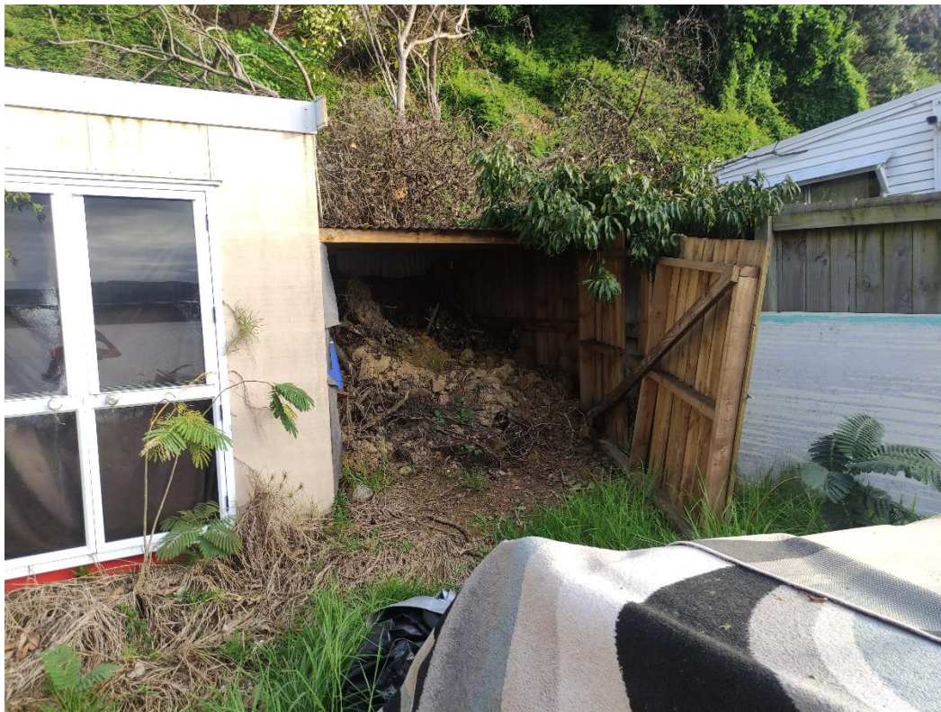
Photograph 14: Damage to shed / car port [REDACTED]
