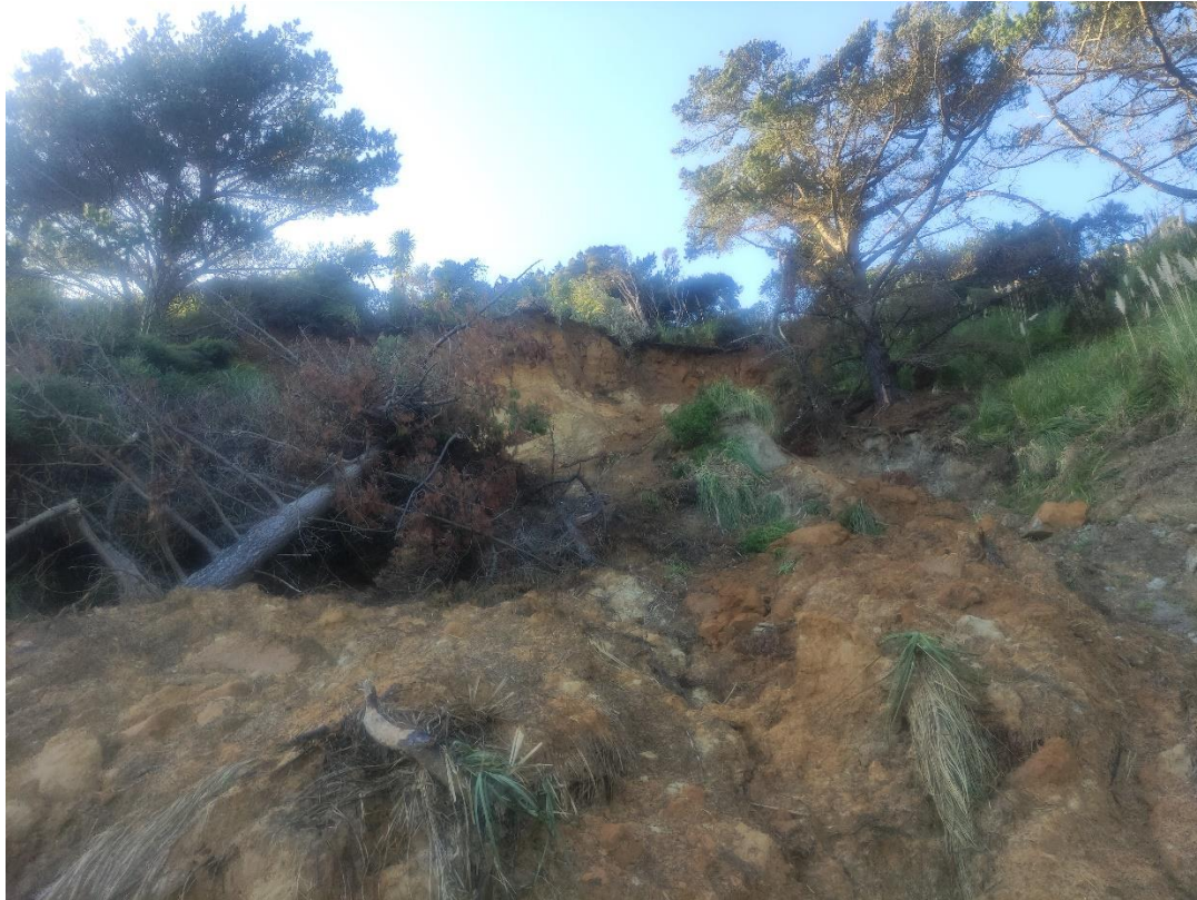
Photograph 5: View of Landslide 5
