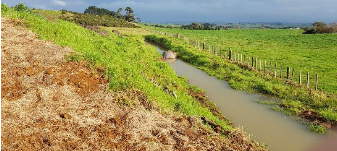
Figure 3: Channel along northern boundary – ponded water spilling across boundary at lower-right of picture. Remove bale and install a series of rock check dams to link to the rock lined channel (see below).
