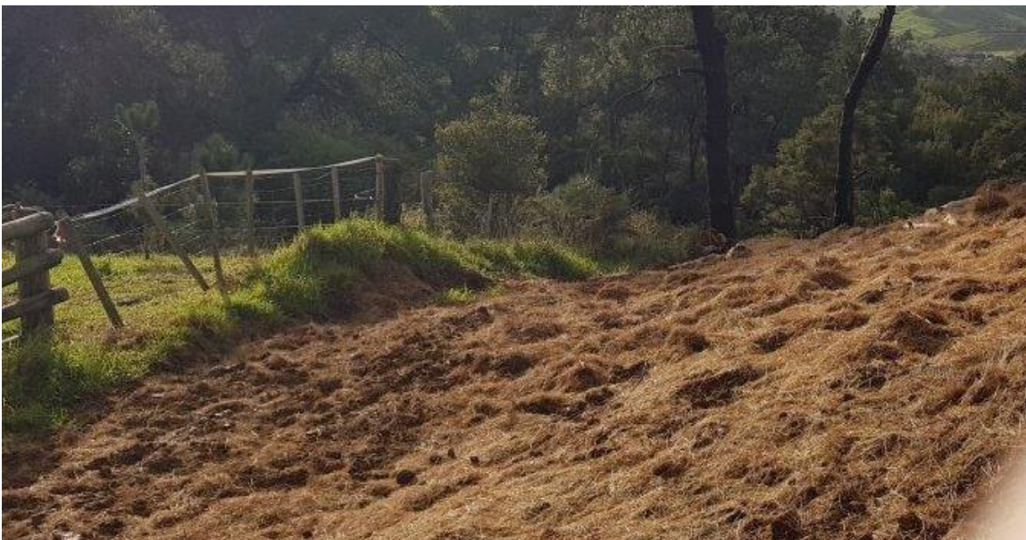
Figure 4: Outlet to east presently blocked with fill and mulched. Install rock lined channel to ensure runoff discharges to a stabilised outfall.
