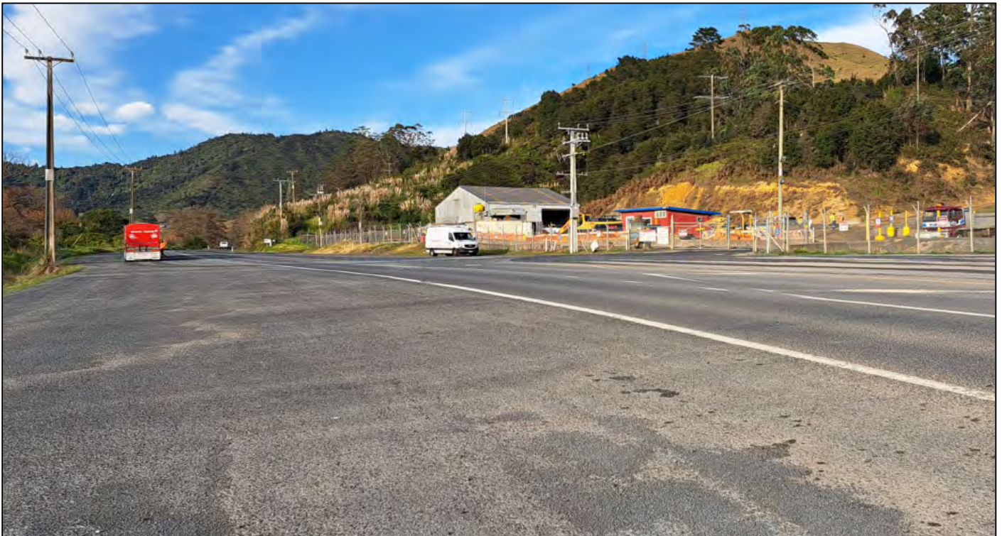
Figure 8: Wide sealed area at the vehicle crossing is used by departing trucks to secure/cover loads etc. There is loose aggregate on the surface. (Photo June 2022)
