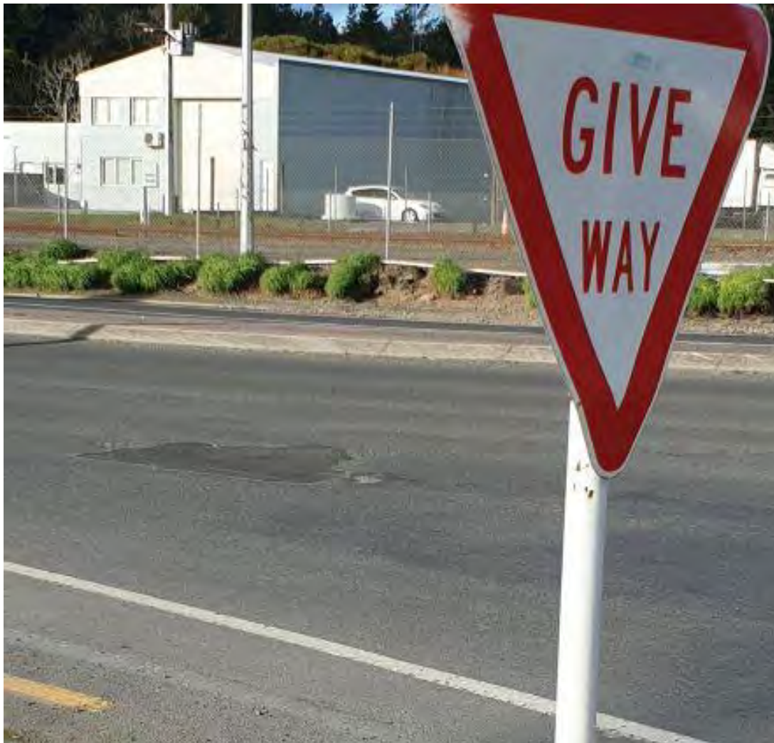
Pothole – a regular at entrance onto North bound lane of Great South Road from Tainui Bridge Road, this is on the merge lane and swerving to avoid it can cause issues
