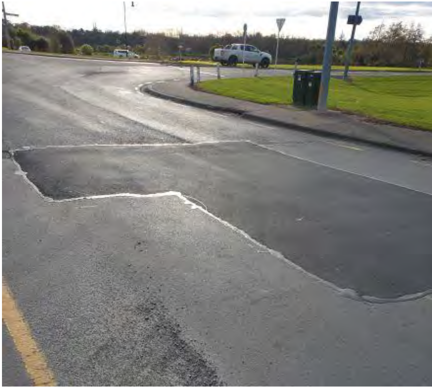
Large Patch from a small pothole – Tainui Bridge Road
