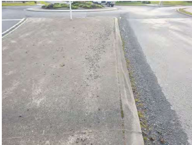
Significant gravel builds up covering road markings, being thrown up onto traffic island
