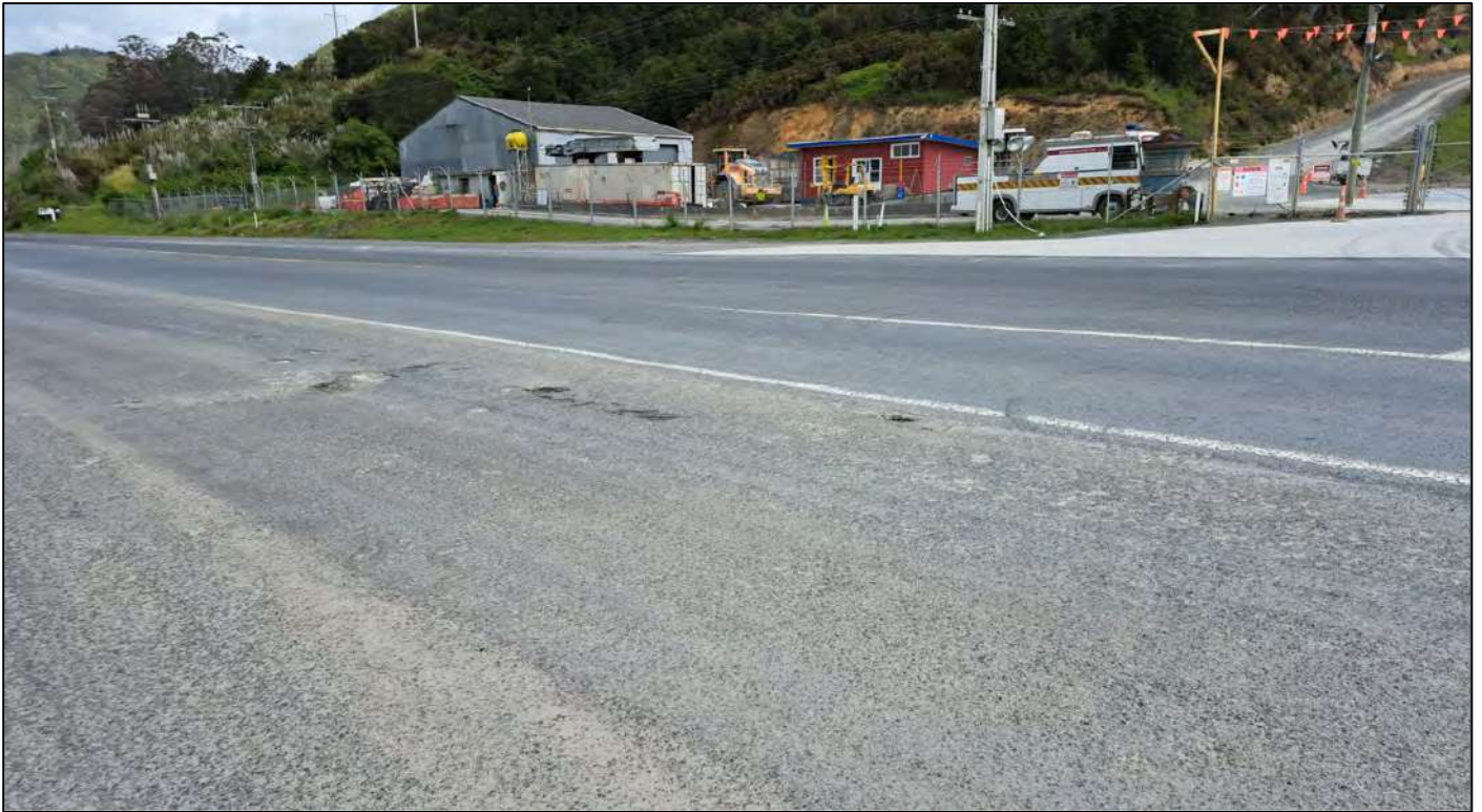
Figure 9: Wide sealed area opposite the vehicle crossing has evidence of potholing. (Photo October 2022)
