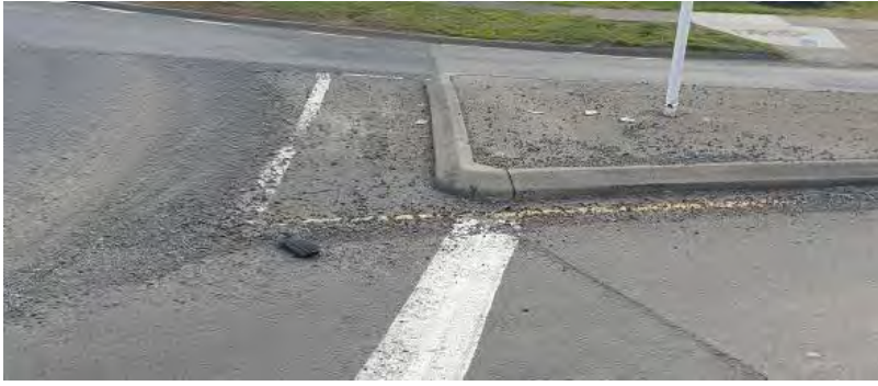
Gravel builds up on and around traffic islands causing a hazard for all users
