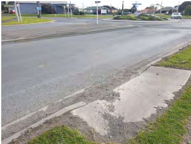
Gravel builds up on pedestrian access, also covering road markings
