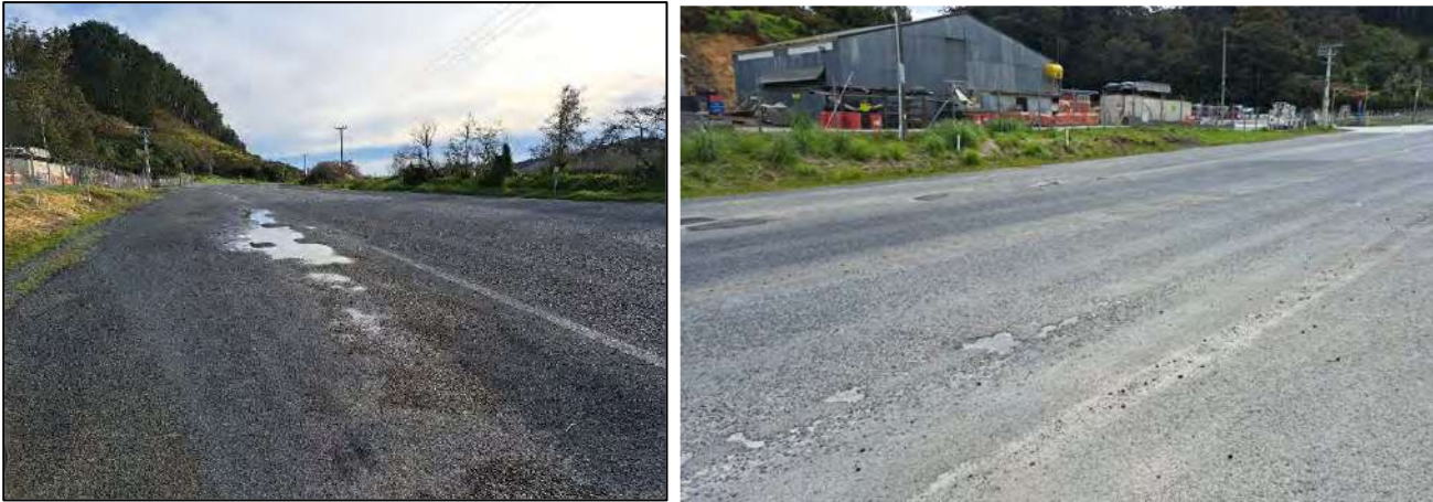
Figure 7: Left turn approach 6m wide sealed shoulder. There is pot holing and evidence of patching. (LHS: June 2022 and RHS: October 2022)
