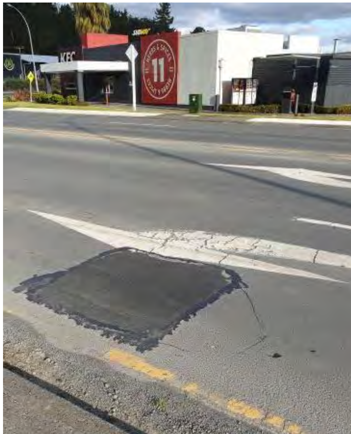
Small patch on Tainui Bridge Road
