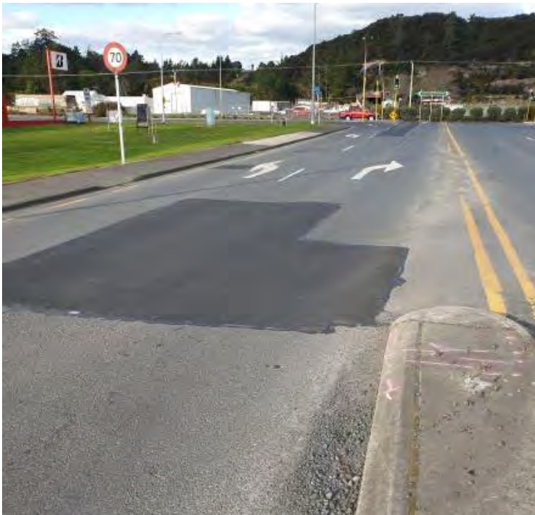
Three patches on road impacted by heavy vehicles, gravel covering road markings
