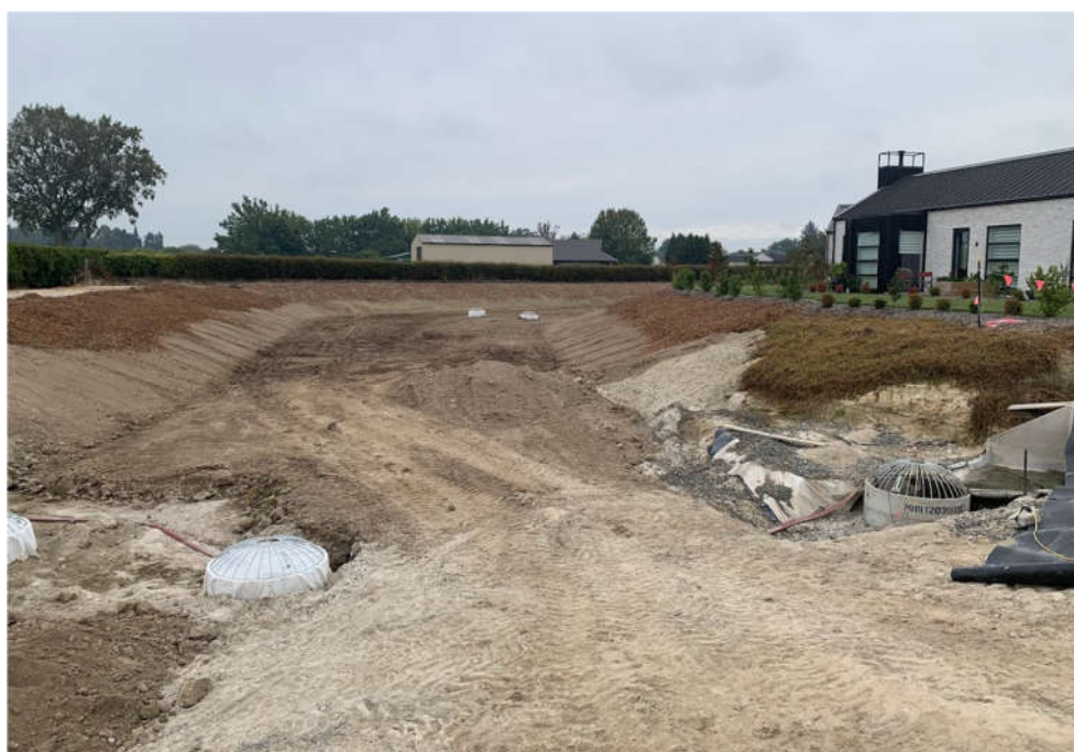
Figure 3: Soakage basin under construction (6 April 2023) – showing scruffy inlets to HYNDS unit prior to pumping first flush to feature ponds.
