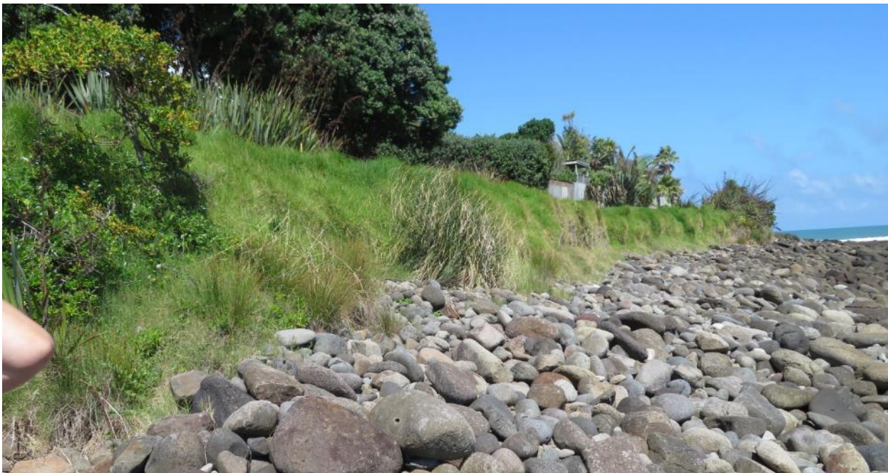
Figure 23: View of vegetated erosion scarp fronting the grassed reserve in Whale Bay township
