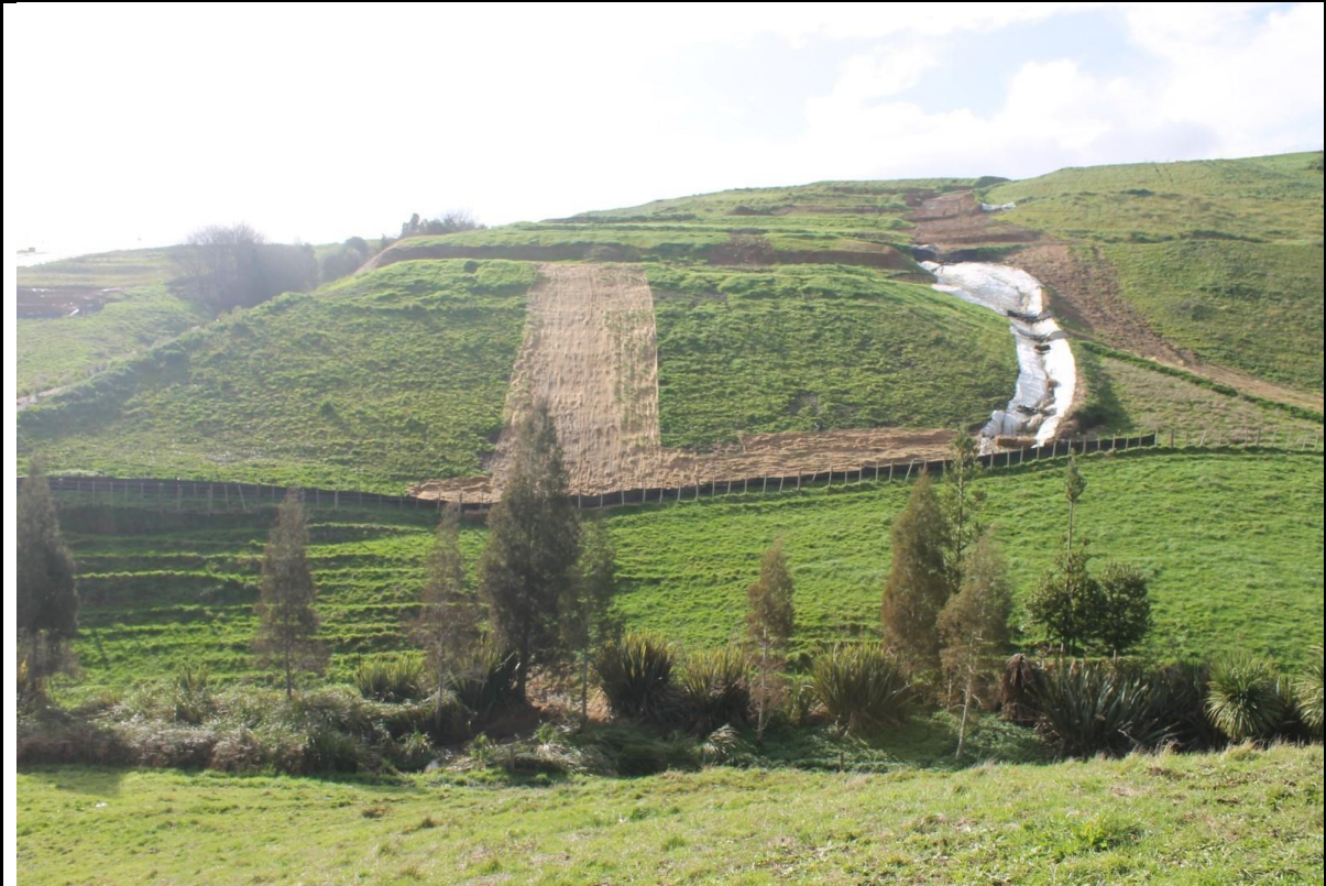
Photo 16. Erosion mitigation middle Dines Stage 5 property (looking north)
