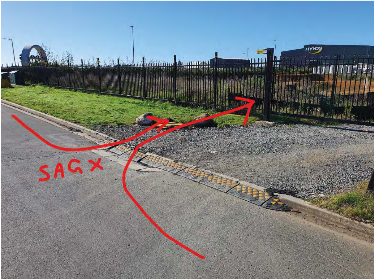
Photo 6 – overland flow enters Hynds site at the road sag.
