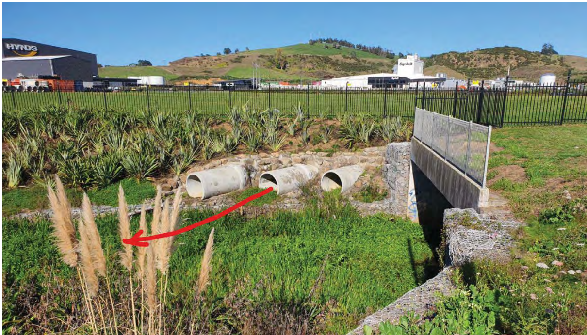
Photo 8 – overland flow discharges to the Tanitewhiora Stream. Completed McDonald Road culvert to the right.
