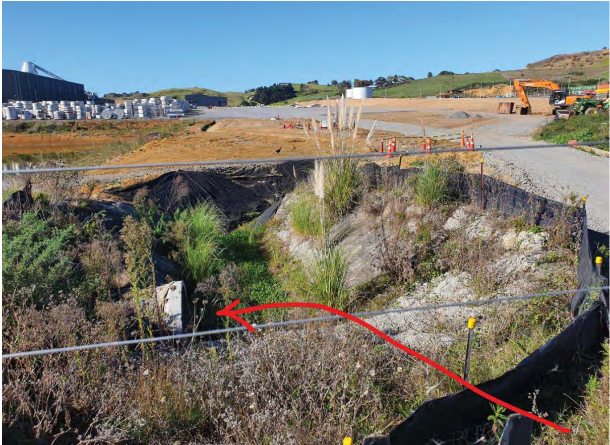
Photo 7 – overland flow from McDonald Road enters the partially complete DN1350 Pipeline A at the road sag/low point
