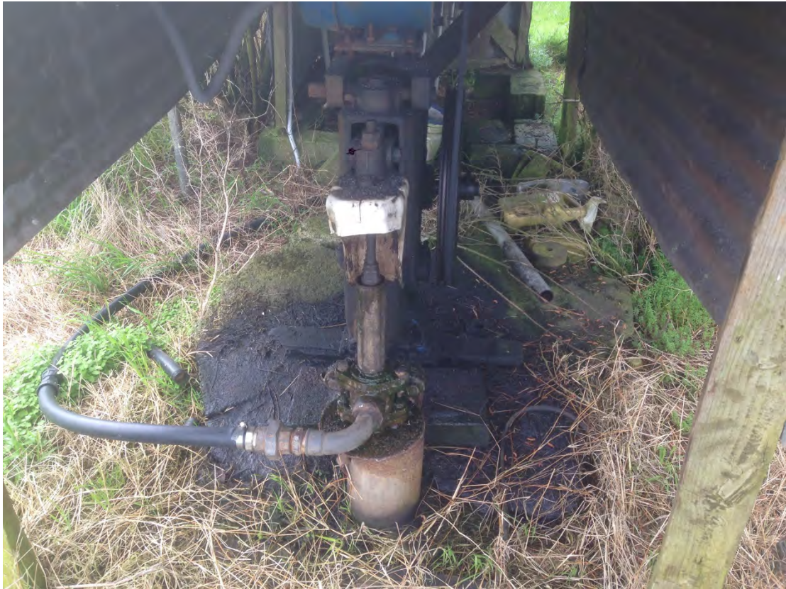
Photograph 3: Close up of farm bore, note staining near pump.
